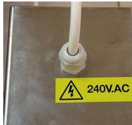
Figure 5. Power cable outlet and Electrical Supply Label.
